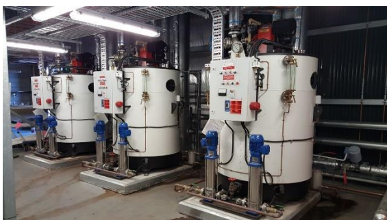
Multi Boiler installation 3 x 500kW, NG fired
